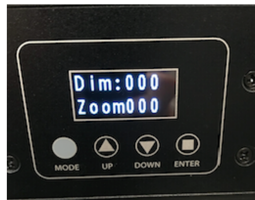
NO DMX CABLE CONNECTED
