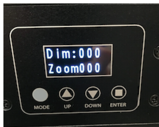
NO DMX CABLE CONNECTED
